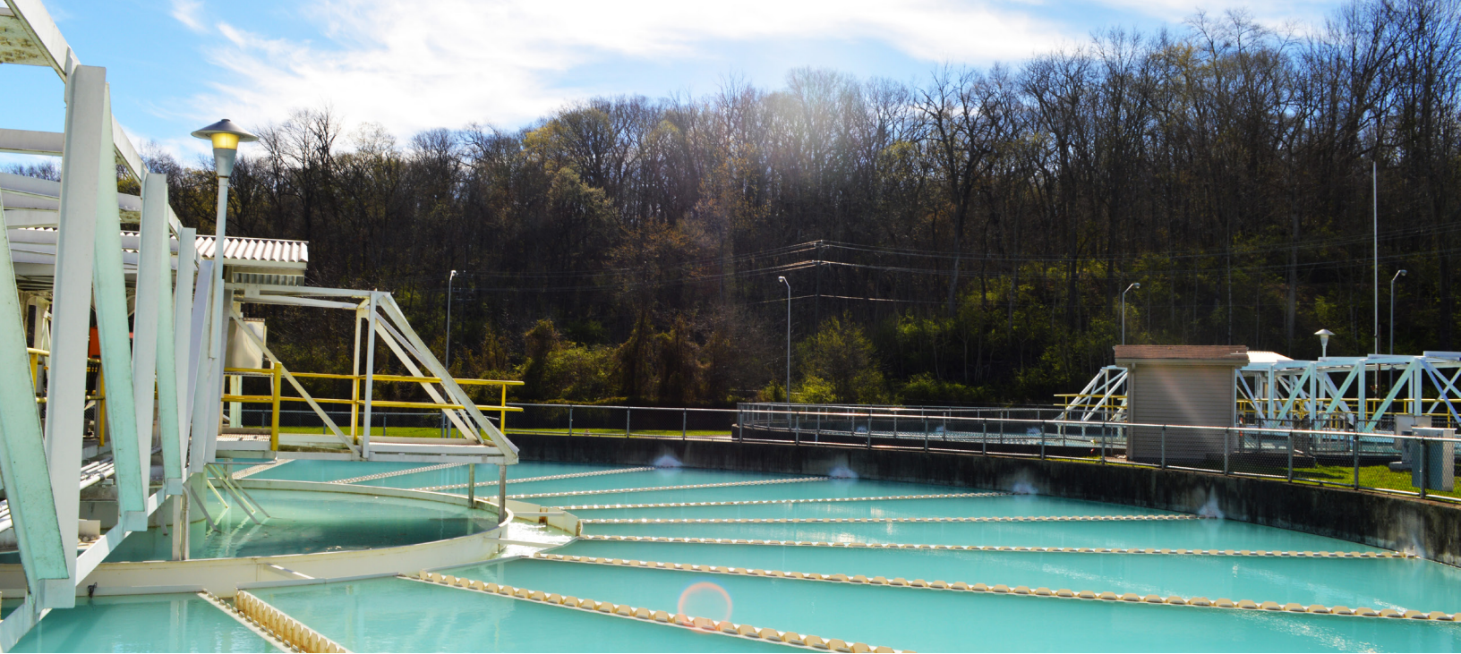
CMBP Solids Contact (Softening) Basins
