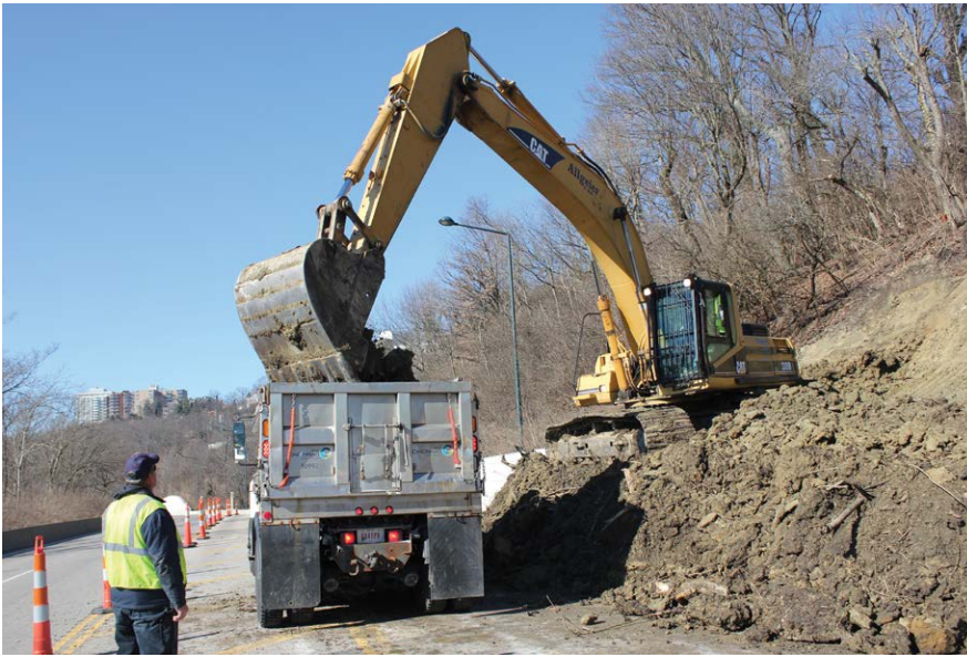
Intense storms caused landslides onto Columbia Parkway in 2016, requiring over $17 million to clean-up and repair. Photo courtesy of City Staff.
