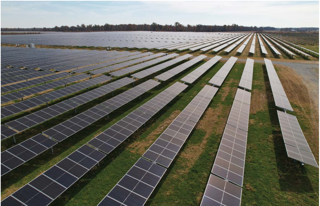
The New Market Solar Array in Highland County provides electricity for City operations and the residential aggregation program. Photo courtesy of Algonquin Power & Utilities Corp.
