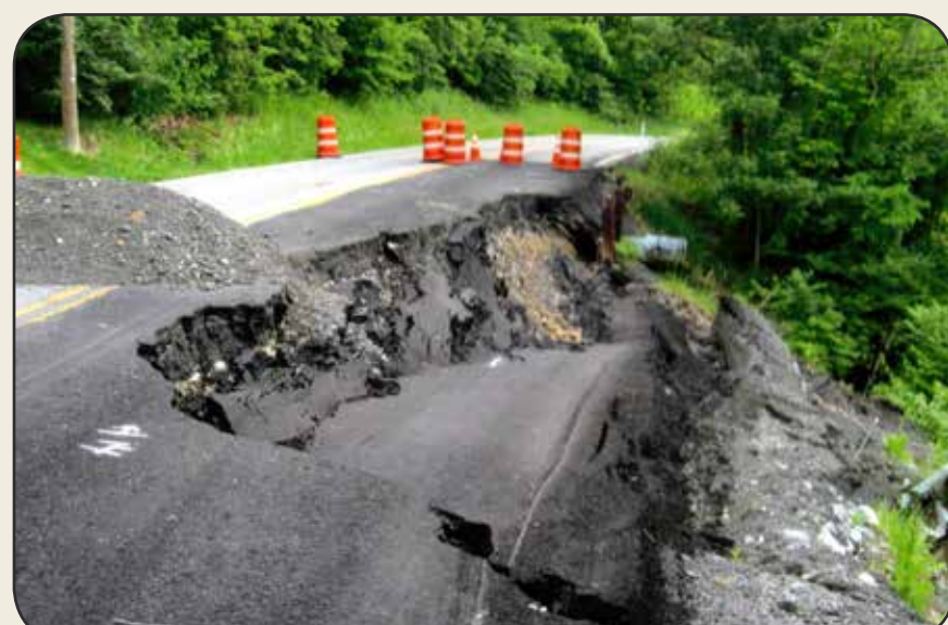
Figure 11. Rotational slide on KY 1486 at Fowler Creek. The fill was placed on top of Kope Formation colluvium, which led to its failure.
