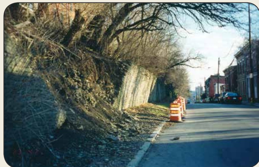
Figure 2. Old, slow hillside creep in colluvium finally breaks this stone retaining wall, in Mt. Auburn, Cincinnati, Ohio. Note the tilted trees.
