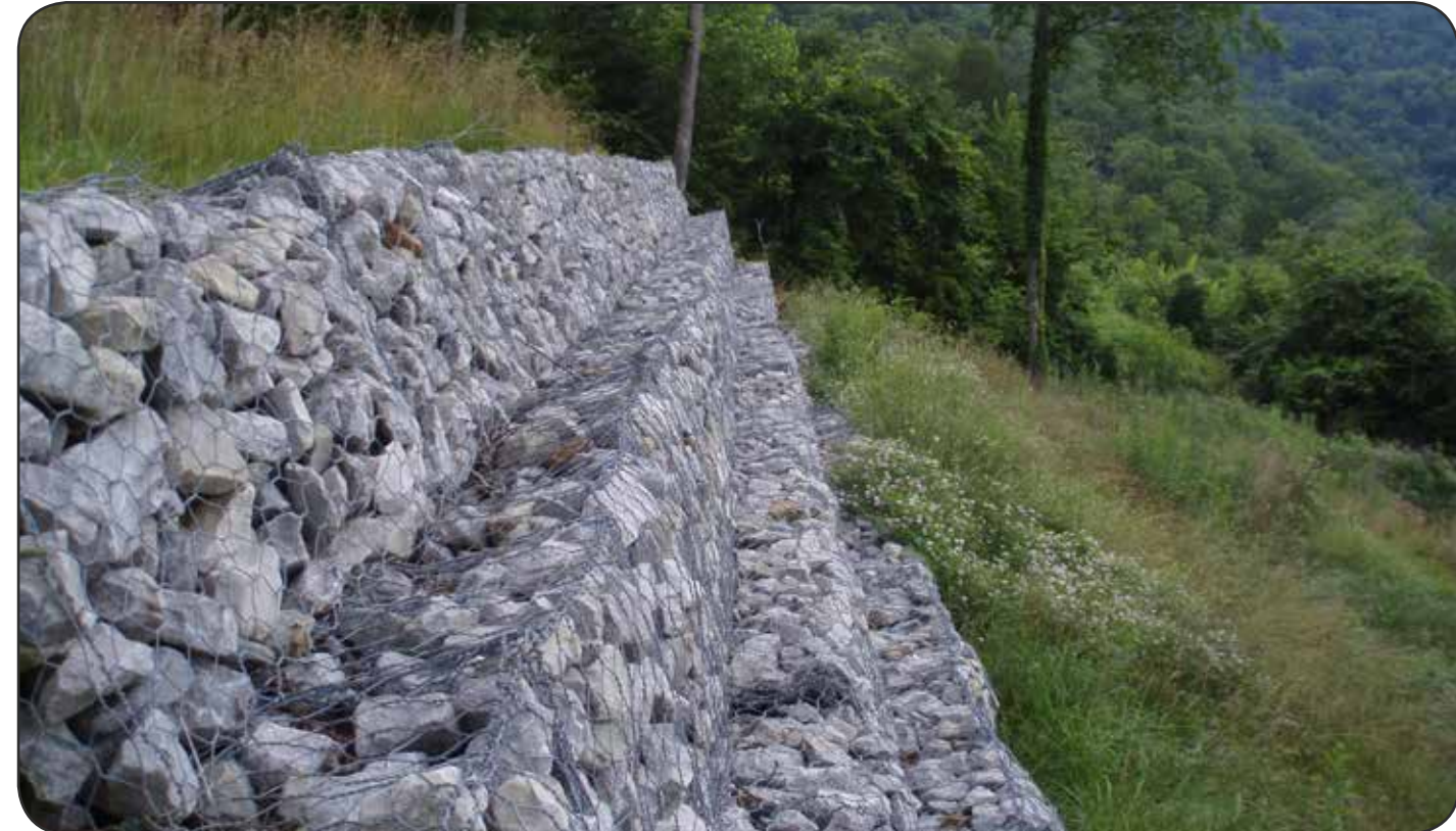
Figure 17. A special caged structure called a gabion wall reinforces a steep slope in Pulaski County, Kentucky.
