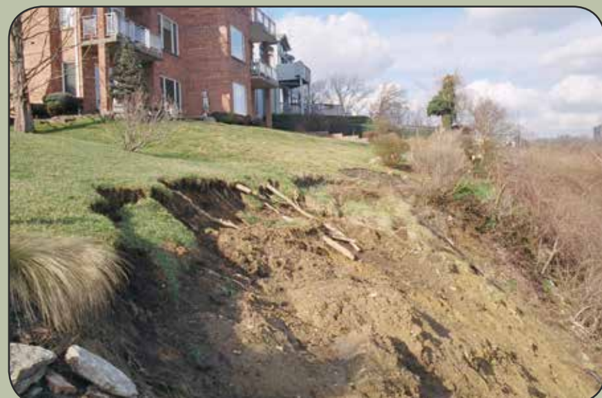
Figure 5. Head scarp of translational slide along the Ohio River Valley, at Price Hill, Cincinnati, Ohio. The apartments are set in bedrock and so are unaffected.
