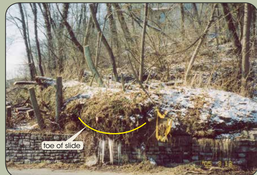
Figure 7. The toe of a translational slide is overtopping a wall. Note the icicles at the base, evidence that water is flowing along the slide surface.
