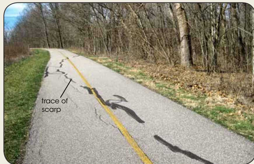
Figure 3. This long curved crack in a walking trail in Miami-Whitewater Park, Hamilton County, Ohio, reveals soil movement towards a stream to the right. This movement would not be readily apparent in a grassy field.
