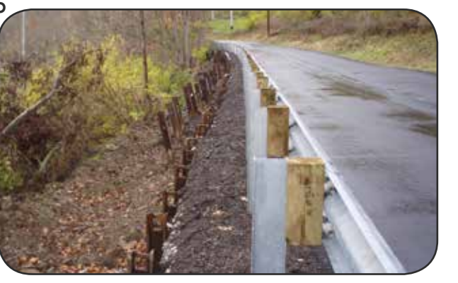
Figure 16b. A retaining wall of steel piles shows generations of failure along a roadway in Kenton County, Kentucky.
