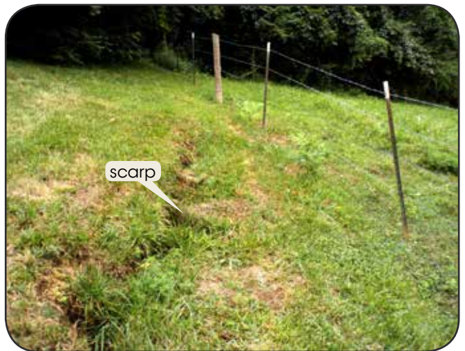
Figure 15. A small, fresh scarp on a gentle slope and tilted fence posts are subtle but important clues that signal sliding. They could easily be missed in dense vegetation.
