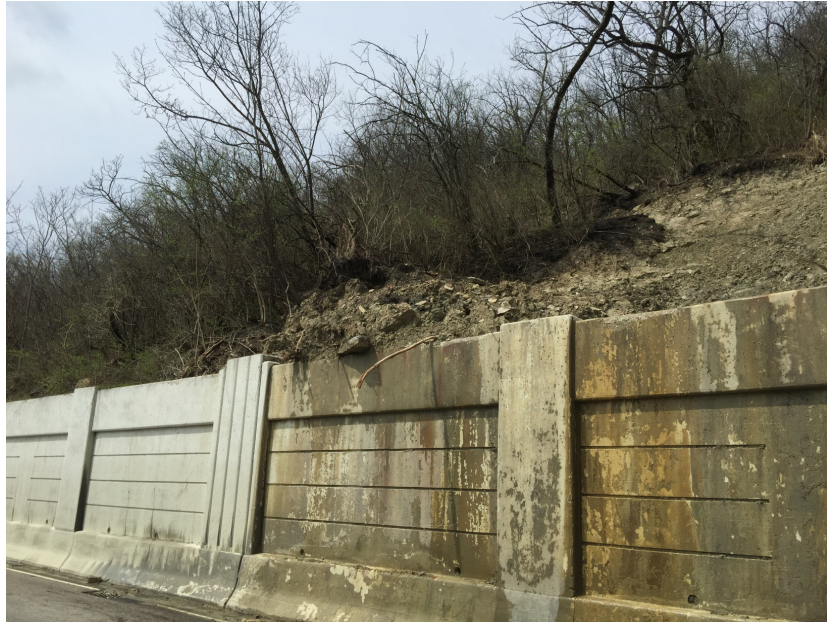
Small debris removed from atop Columbia Parkway Wall.
