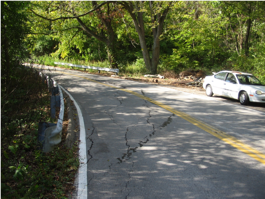
Hillside Avenue east of Tyler. Note sealing of tension cracks in roadway.
