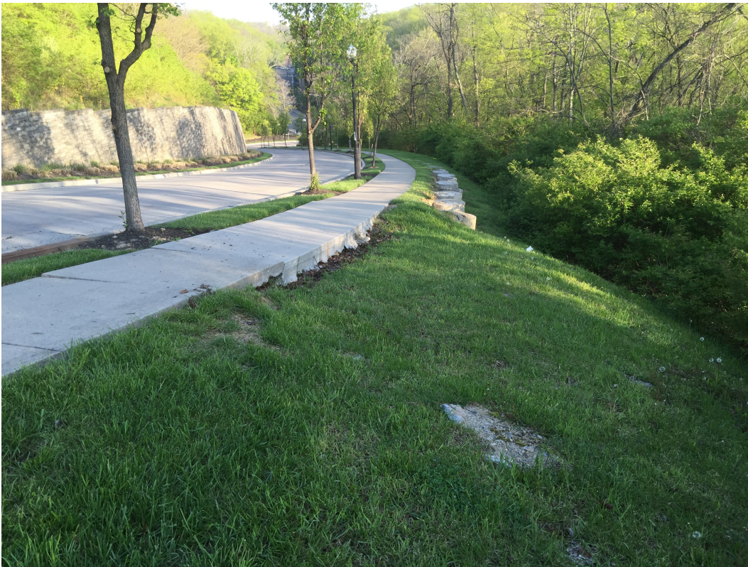
Ridgetop Way looking towards Queen City Avenue showing existing wall and undermining of sidewalk. Headscarp of landslide extends into the forward lawn area.
