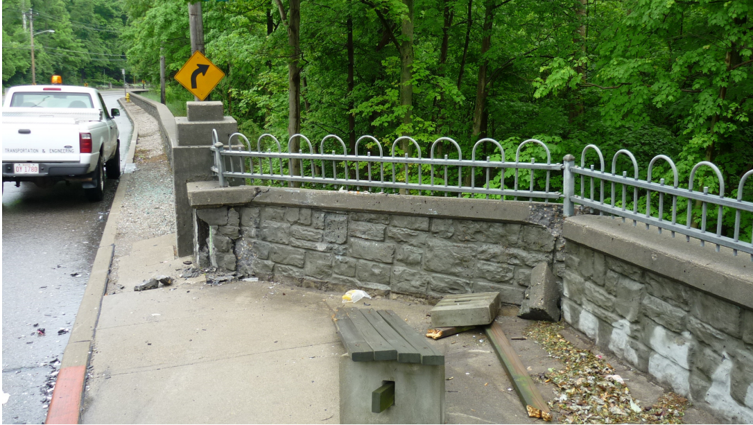
Damaged Colerain Avenue retaining wall opposite Raeburn Drive.
