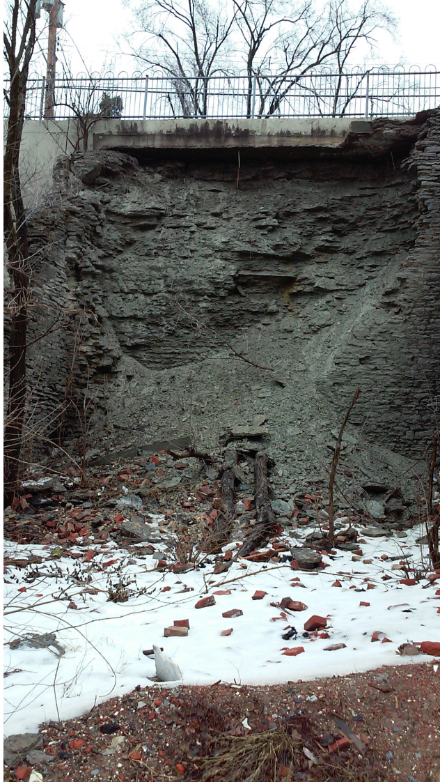
View of Dorchester Avenue from below on Sycamore Avenue. Note undermining of Dorchester wall cap and sidewalk. Shale and limestone bedrock exposed in face of slope.
