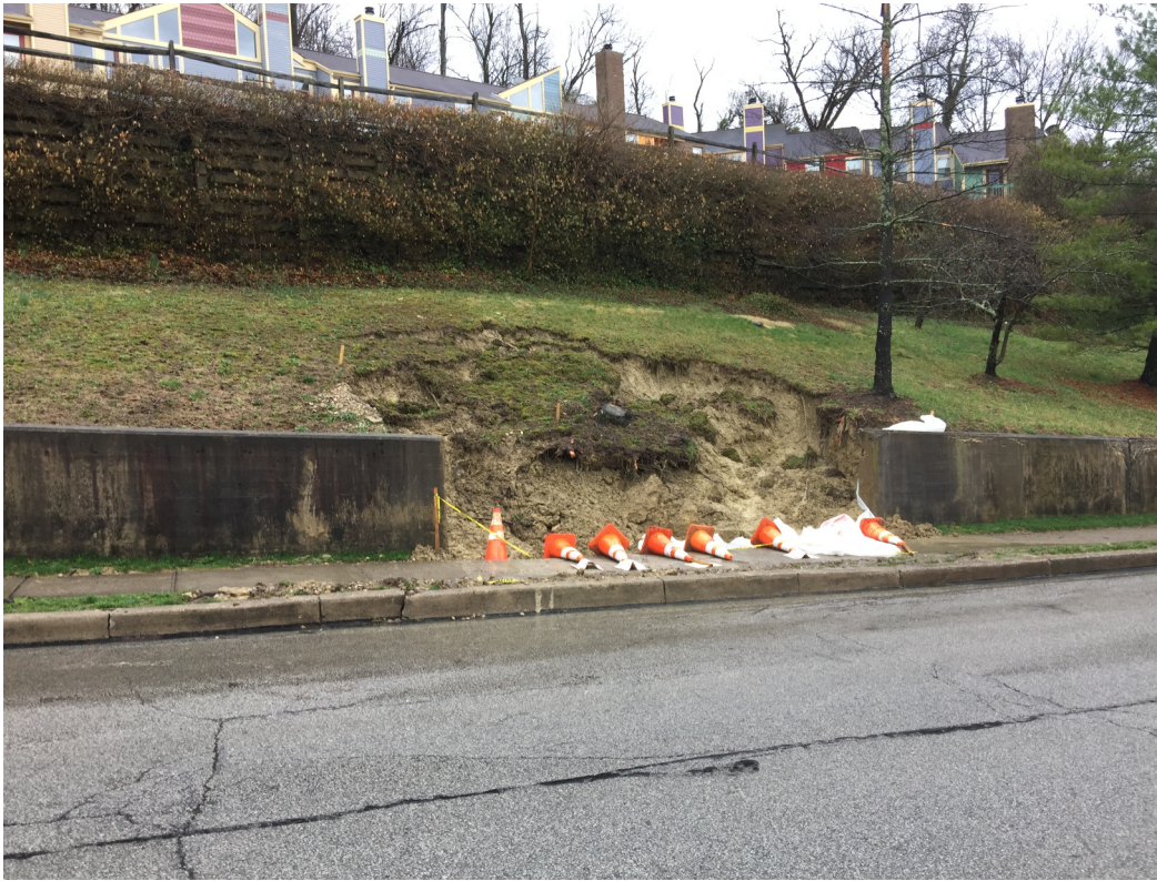
Tusculum Avenue after wall failure. Failed wall stem has been removed.
