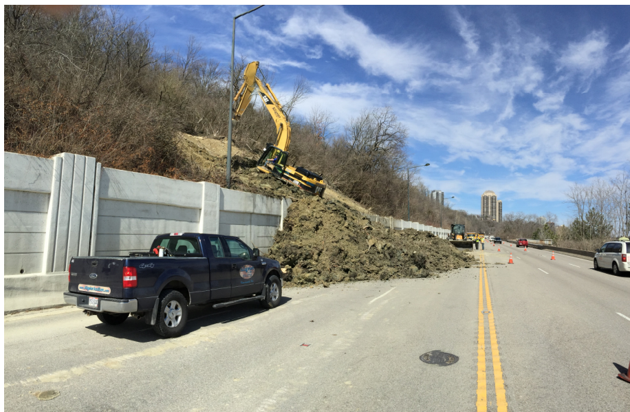
Removal of slide debris from Columbia Parkway approximately 2,000 feet west of Kemper Lane.
