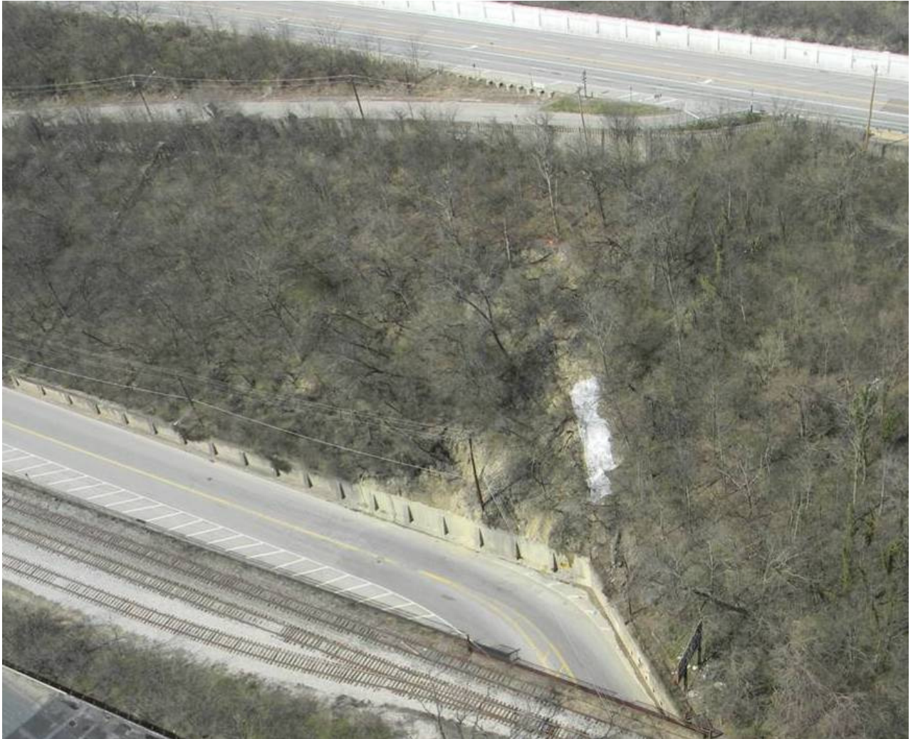
Aerial view of landslide on Riverside Drive west of the Rookwood Overpass. The property above the wall is owned by the Park Board. Note extent of headscarp. Plastic sheet left behind after test pits were dug in 2011 to prevent water from seeping along scarp line into the slide mass. Plastic has since deteriorated and no longer exists.
