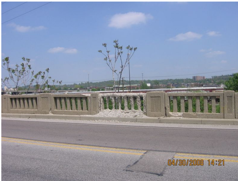
Disintegration of railing exposing steel reinforcement most likely due to salt spray.
