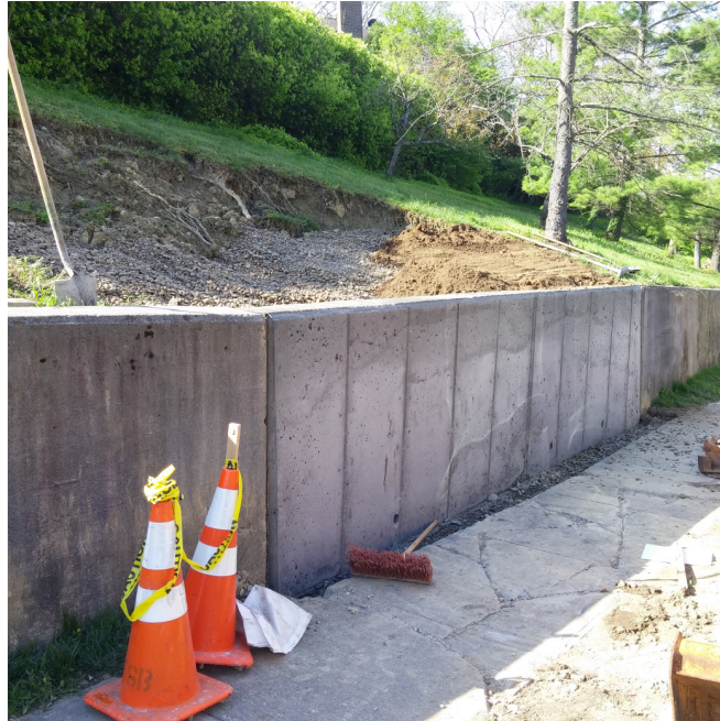
Tusculum Avenue after completion of wall stem and prior to backfilling and sidewalk replacement.
