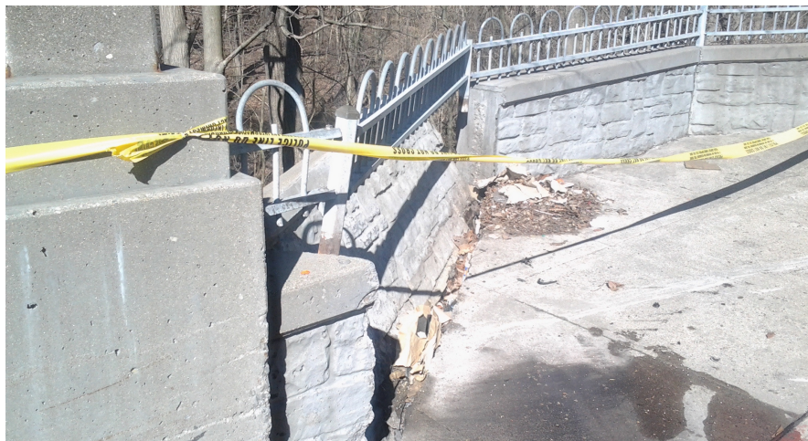
Damaged Colerain Avenue retaining wall opposite Tranquility Lane.
