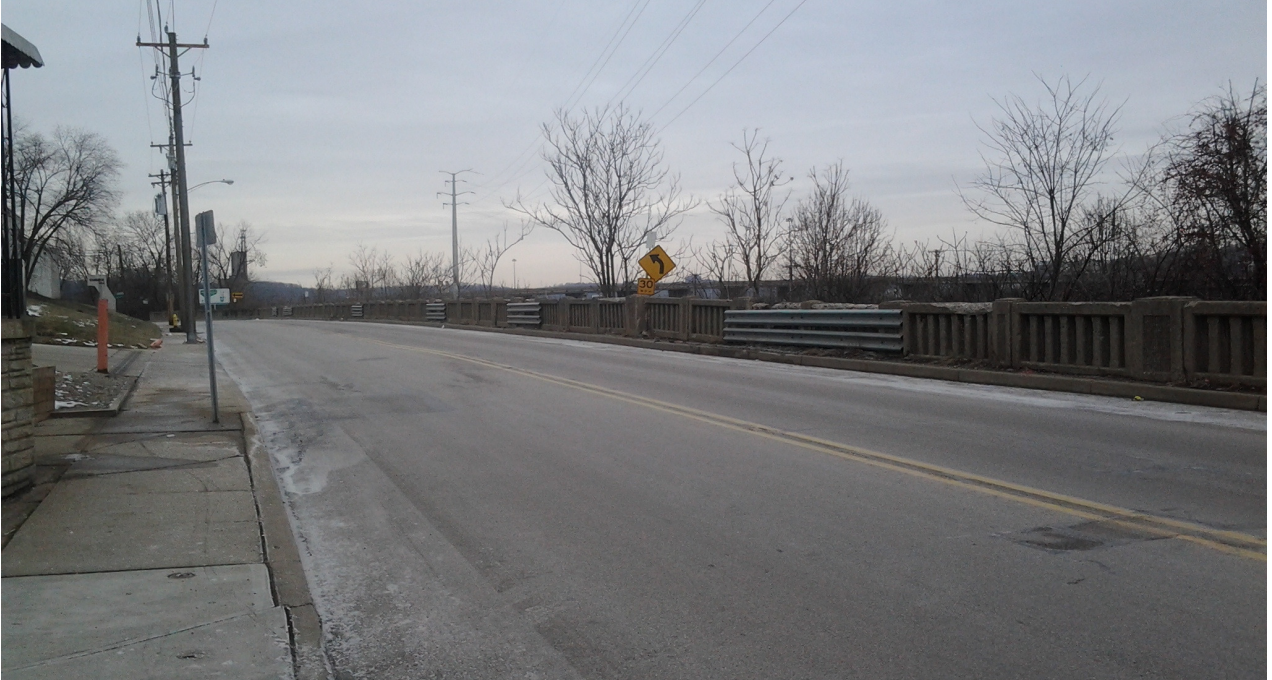
Sections of concrete railing replaced with guardrail sections bolted to pilasters on Cummins Street.
